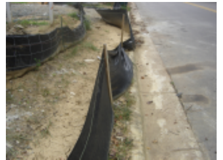
The silt fence shown above, referred to as "silt fence on a stick", is not approved as an erosion control device by the Wake County Erosion Control Ordinance.
