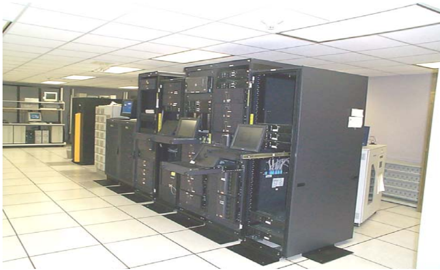
Storage Area Network (SAN)
