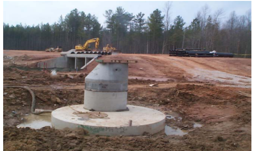
Water Sewer Infrastructure
