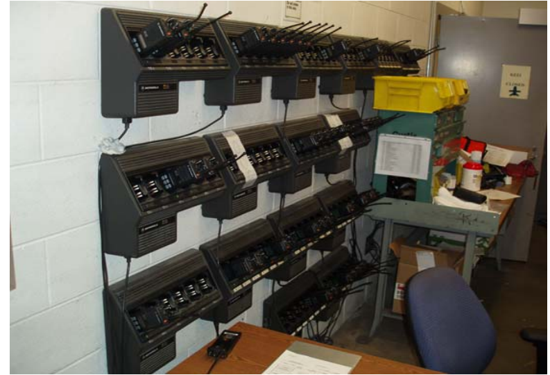
800 MHz Radio Recharging Station
