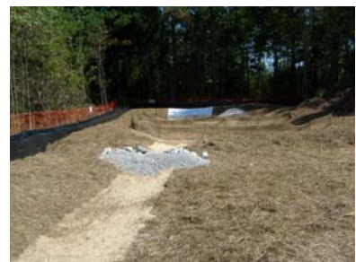
Inlet Protection into Custom Basin
