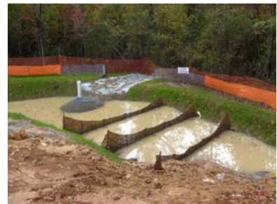
Custom Basin with Porous Baffles and Vegetated Inside Slopes
