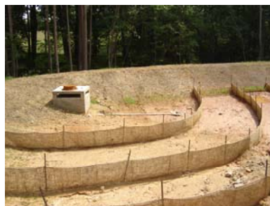
Skimmer Sediment Basin with Porous Baffles
